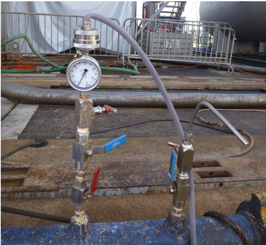
Figure 8: Filtering device at drillsite Honselersdijk consisting of ball values, feed regulator, pressure gauge and a cross flow sampler on top.
