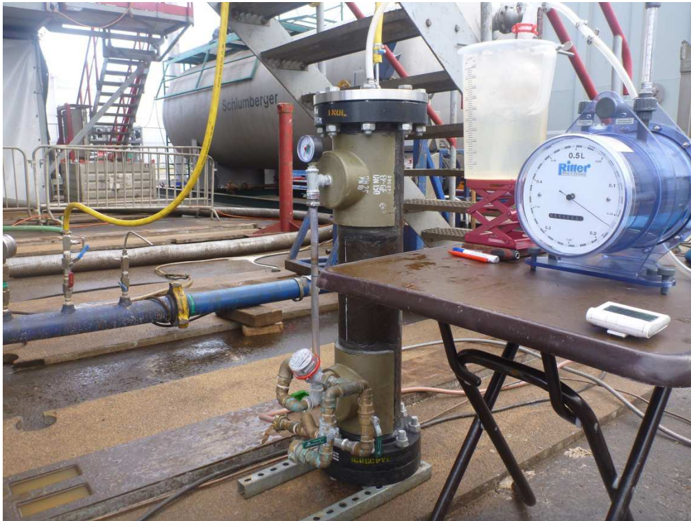
Figure 1: Degasser at the well Honselersdijk Gt 1
