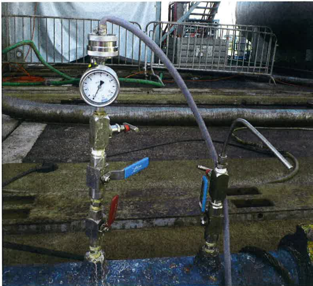
Figure 8: Filtering device at drillsite Honselersdijk consisting of ball valves, feed regulator, pressure gauge and a cross flow sampler on top.
