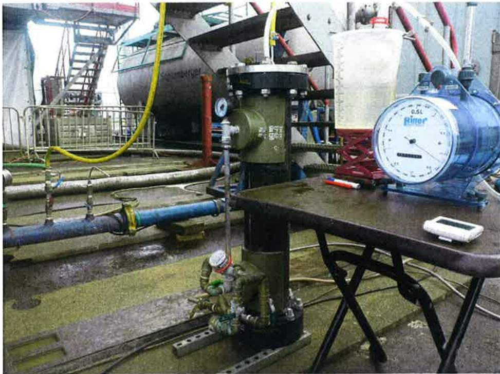
Figure 1: Degasser on the well Honselersdijk Gt 1
