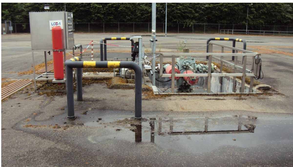
Figuur 11-4: Foto wellhead put WWS-01.
